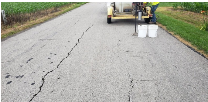
Existing Pavement Condition along Jackson Road, cracking throughout the project included longitudinal and block cracking
