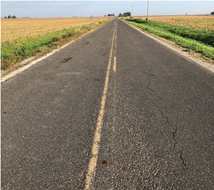
Original Narrow, Distressed Pavement
