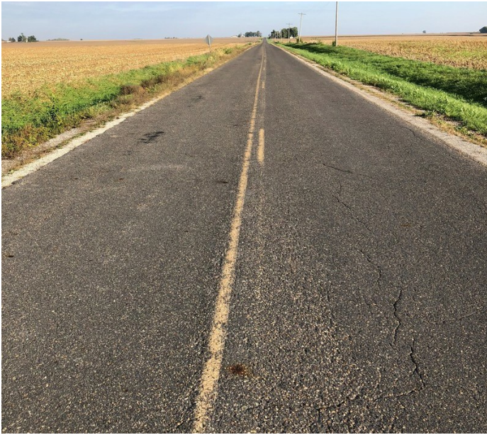
Original Narrow, Distressed Pavement
