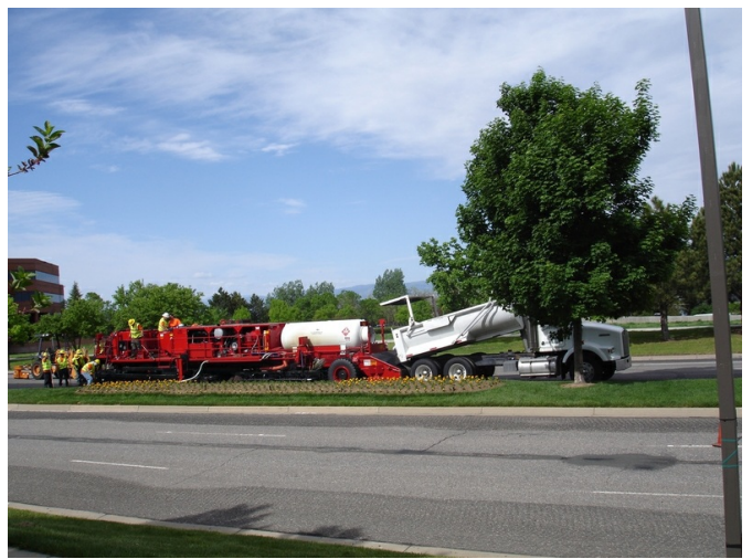
New hot mix asphalt produced in Denver's own hot mix plant is delivered to the Cutler Repaving equipment.
