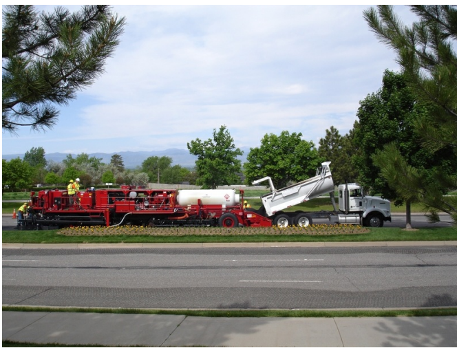
Cutler Repaving's single pass recycling process completes the recycling and resurfacing simultaneously, thereby minimizing delay and inconvenience to the traveling public.
