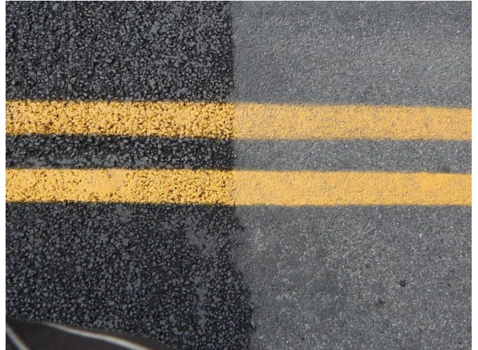
Finished Surface comparison - fiber reinforced interlayer with chip finish on right / PPST Overlay Finish on left
