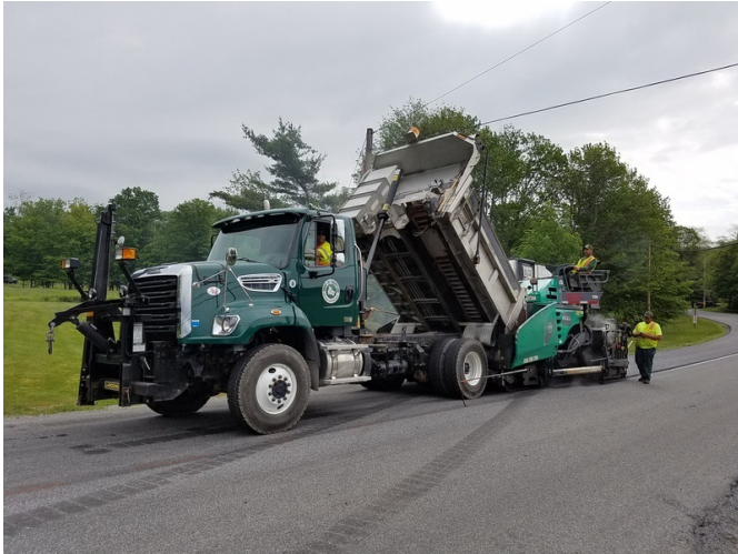
The Gorman Group paving with PPST Type B, utilizing the Town of Thompson to haul material
