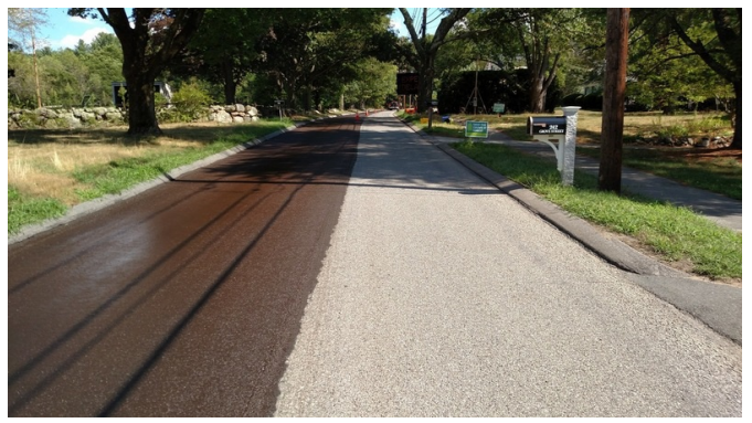
Micro surfacing over chipseal on one side and chipseal on other side of roadway
