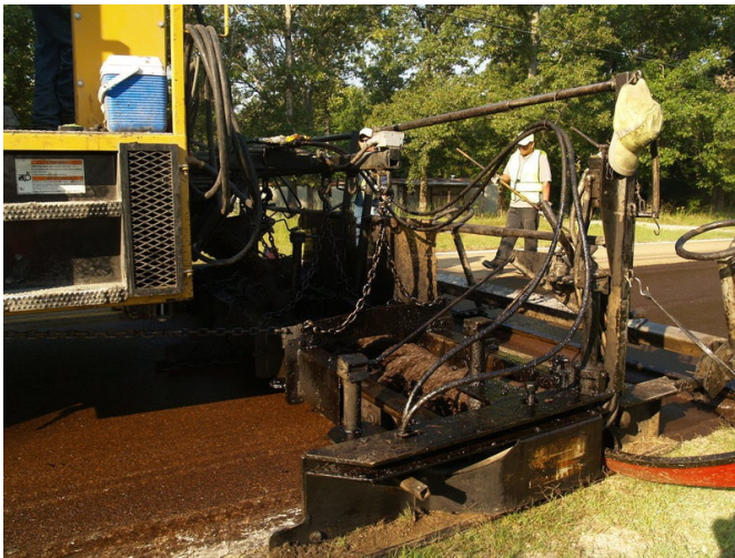
Micro surfacing is placed at the rate of about 22 pounds per square yard to produce a surface treatment between 3/8-inch and 1/2-inch thick.
