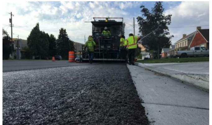
Micro Surfacing Application by Intermountain Slurry Seal with Bergkamp M1E Continuous Paver
