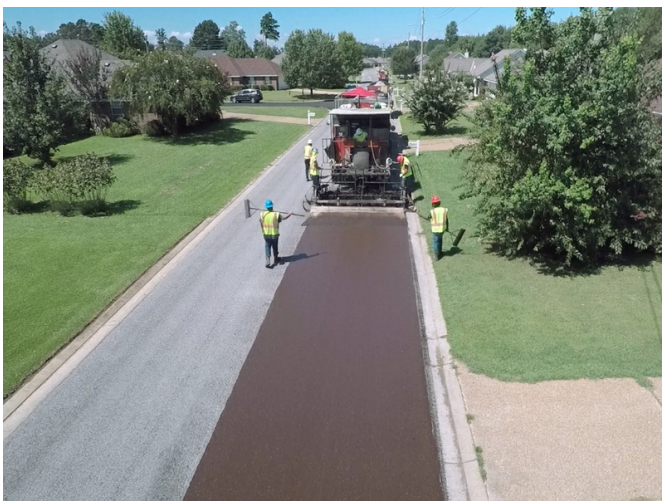
Chip Seal and Microsurfacing was applied to this neighborhood in Rankin County
