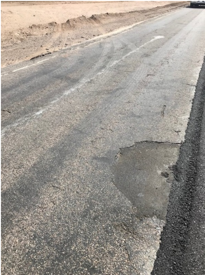
Existing Condition/ some patching
