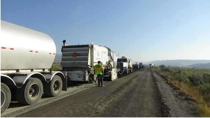
Juntura Cutoff with Portland Cement spread ready to be put in the mix
